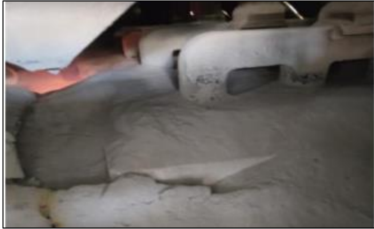
Figure 4. Coated anode condition (1 week old).
